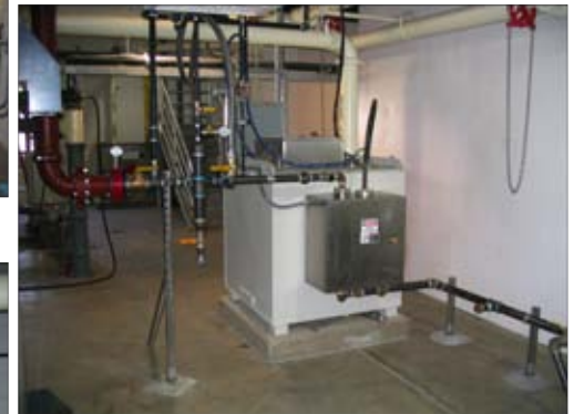
Modulator and treatment chamber
