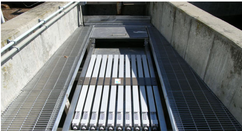
UV unit outdoors – Photo Courtesy of Trojan Inc.
