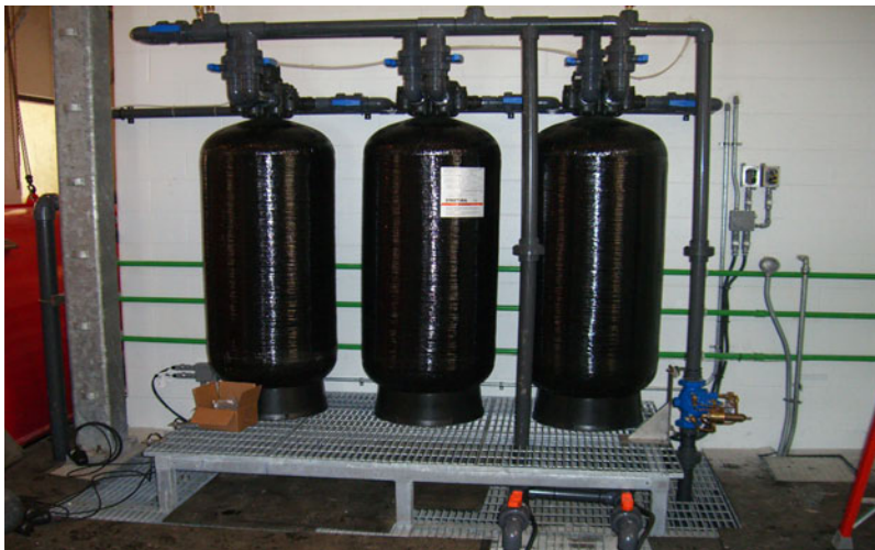
Snow Valley Ski Hill WWTP – Pressure Filters
