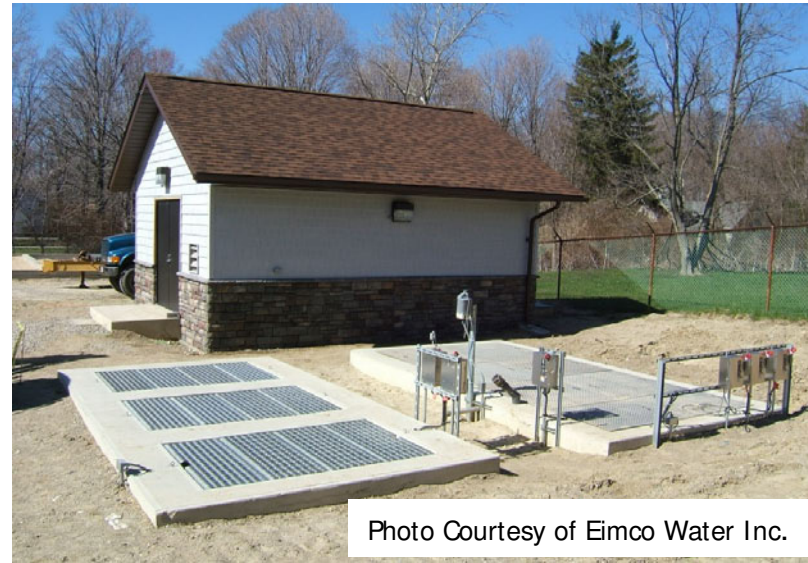
PRE-ENGINEERED PLANT (usually up to 3800m 3 /day) Poured In Place Concrete Tanks
